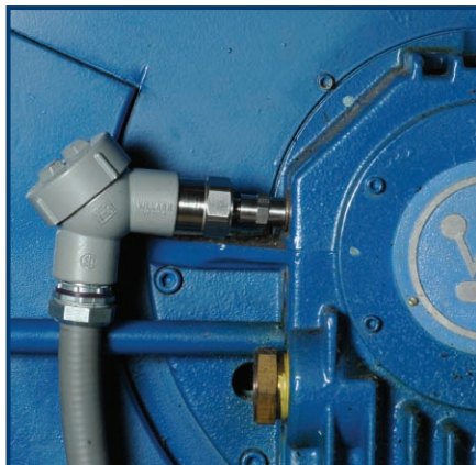
Bearing vibration monitoring on an electric motor
