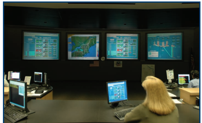
Vibration levels are monitored at the control room
