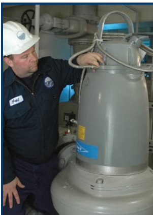
Vibration transmitters monitor vertical pumps in a water treatment facility
