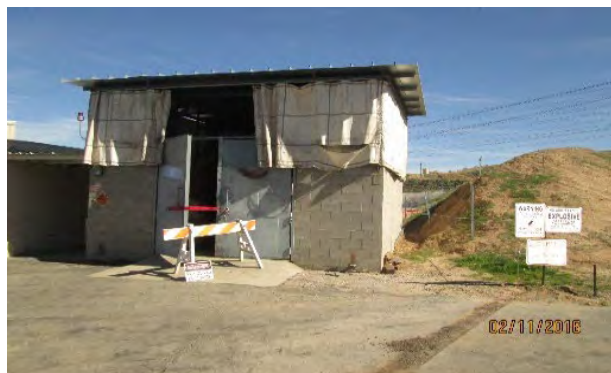
Figure 3A. Hardened Instrumentation Room
