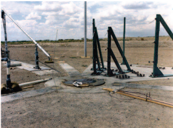
A typical blast sensor installation requires long cables for signal transmission. Data acquisition equipment may be thousands of feet away.
