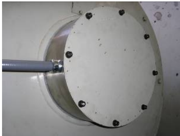
Figure 6 Diode Wheel Inspection Hatch Extension For Additional Clearance
