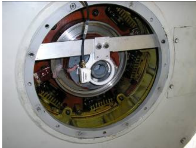
Figure 5 Mounted Adaptor Plate, Transmitter & Receiver Antenna
