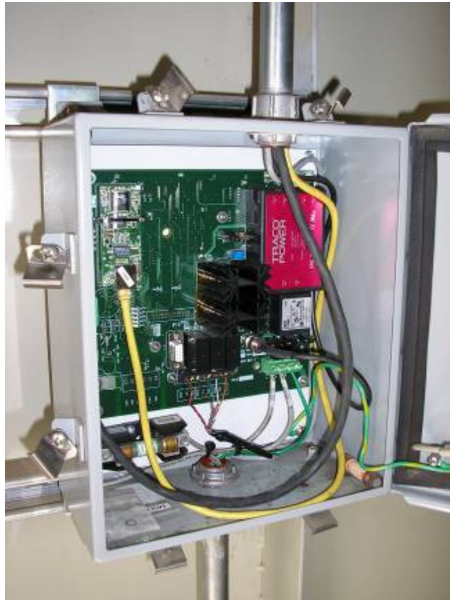
Figure 7 EFREM Receiver Mounted on Exciter Cubicle Wall
